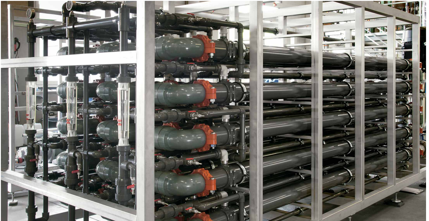
Reverse osmosis plant for the low- and mid-pressure part of ZLD.eco 2
