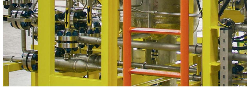
Hydrocyclone pipe spools
