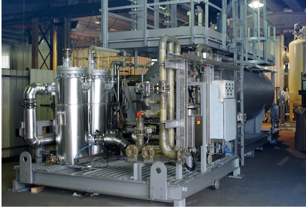
Solids filters and package controls
