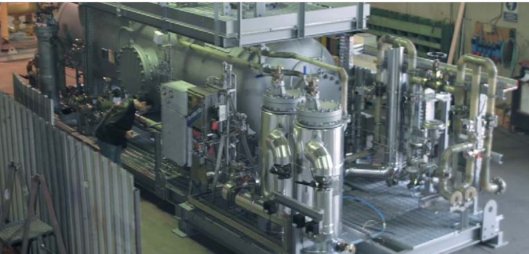
Coalescing filter, CPI and solids filters (left to right)
